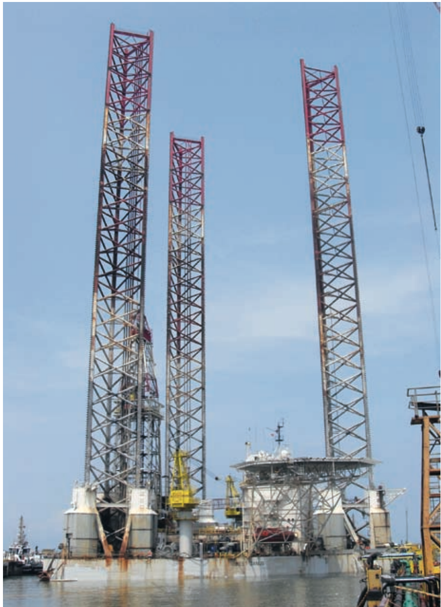
Keppel FELS was commended by Seadrill for the repair and upgrading of West Janus
