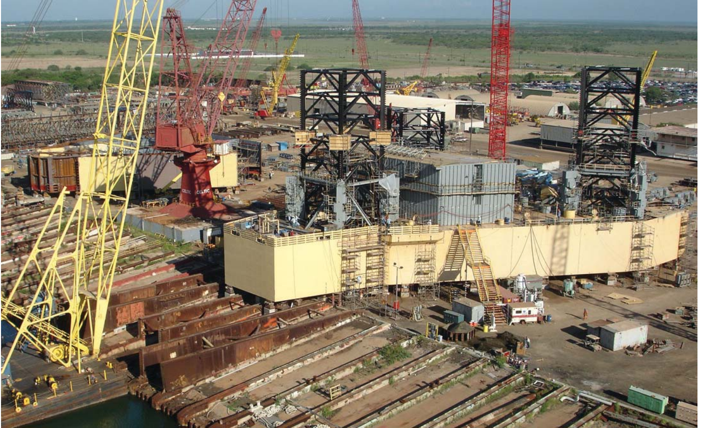
Offshore Courageous (front) and Offshore Defender are two of the five jackups Keppel AmFELS is building for Scorpion Drilling
