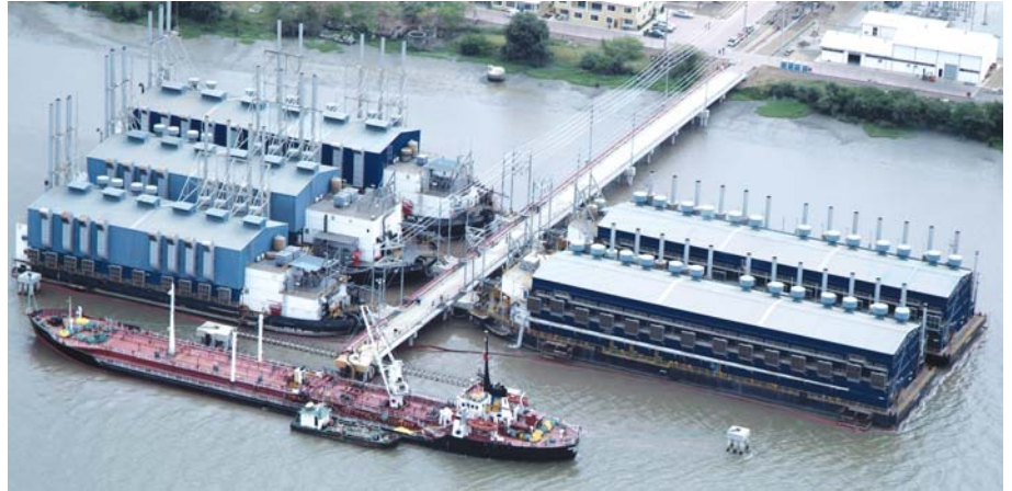
Keppel Energy's power barges will support the rising power demand in Ecuador
