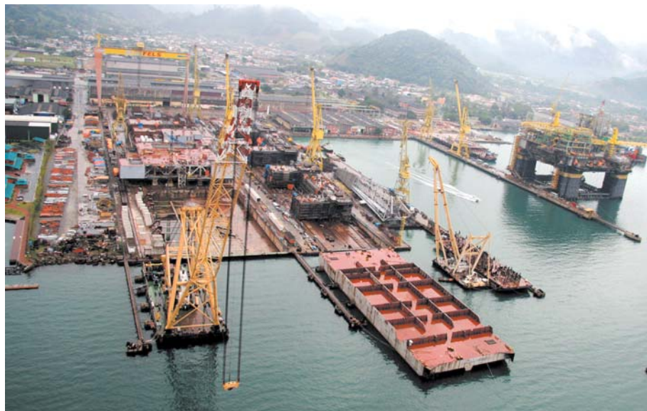
The BrasFELS yard bustling with activity while delivering quality products and services
