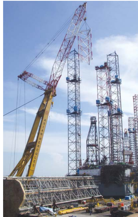
One of the key facilities that Keppel has invested to build up its rig construction capabilities is the floating cranes
